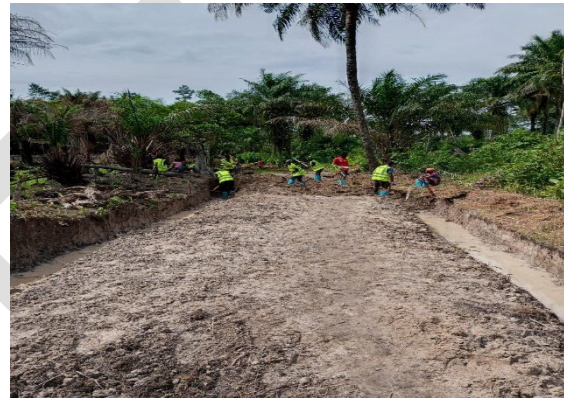
Figure 1: Building Village Access Roads in Lofa. Photo credit: Liberian-Swedish Feeder Roads Project (LSFRP)
